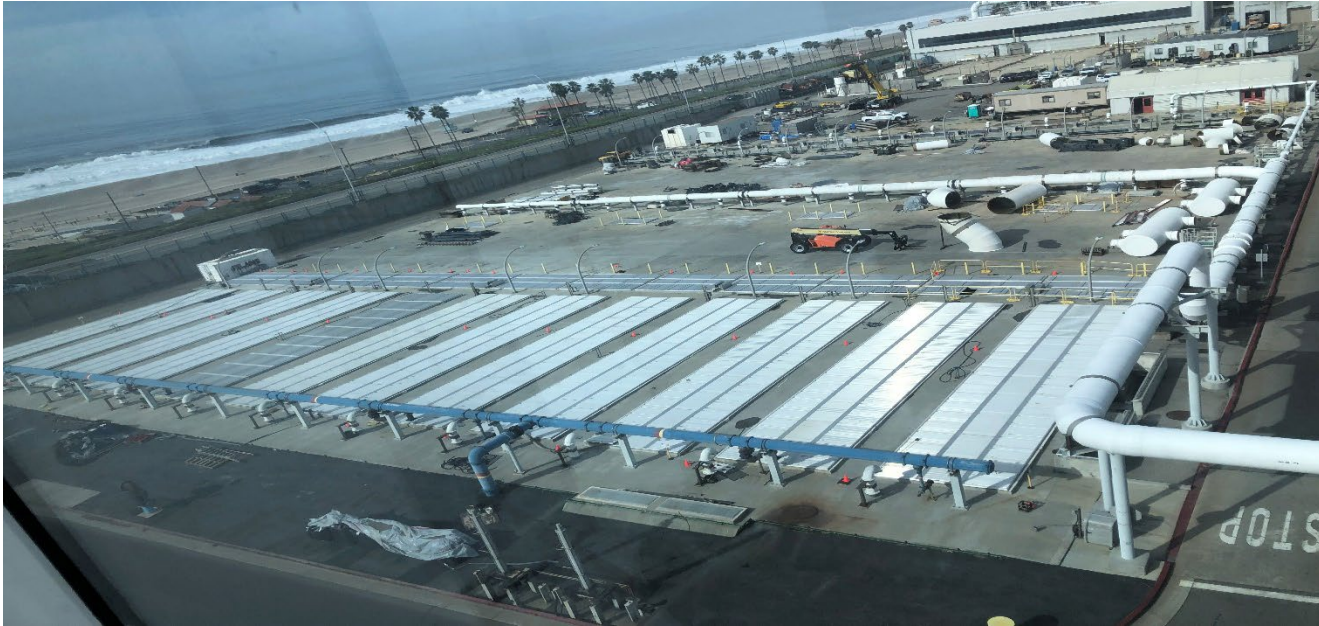
REFURNISHED PRIMARY BATTERY A TANKS
