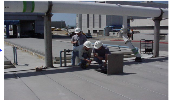
REPLACE TANK COVERS
