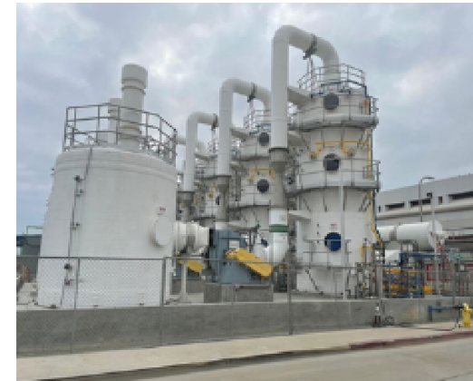
Intermediate Pumping Station BTF
