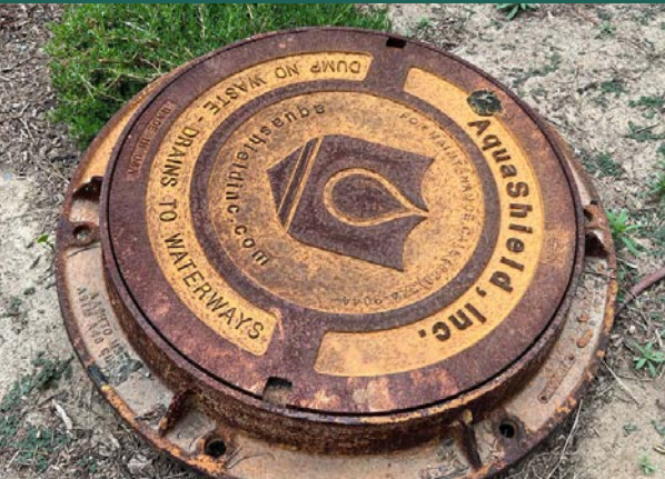
Stormwater treatment device.
